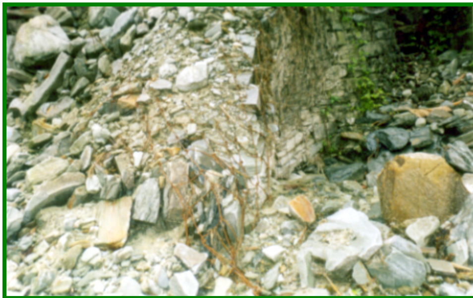
Damaged wall due to over flood within landslide and portion has been protected
