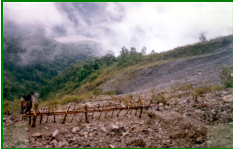
Bally benching in the landslide to arrest the soil erosion and vegetation regeneration
